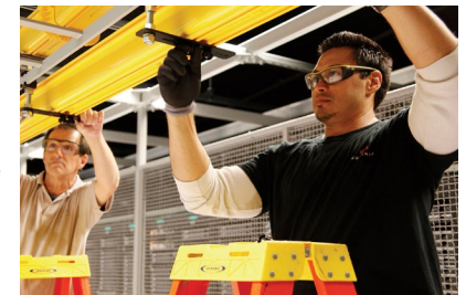
Equinix IBX data center technician
